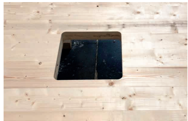
Cut-out, residual radii not removed
